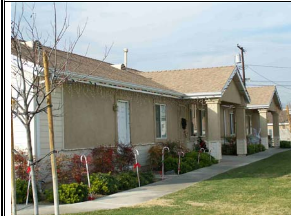
Figure 36: View looking northwest at a highly modified former barracks, which has retained its original length. Building is located at 8371 Janet Avenue
