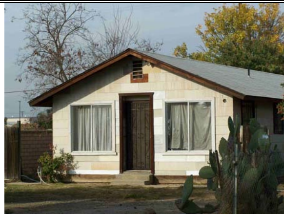
Figure 27: View looking northwest at the post-war era asbestos asphalt shingle cladding and replaced windows of 7771 Janet Avenue
